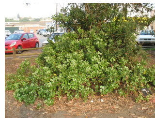
BEFORE: Tree growing through the tar in one of the parking bays
